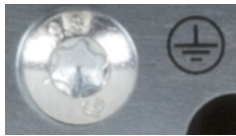
Figure 7-13 Bonding Ground Connection
